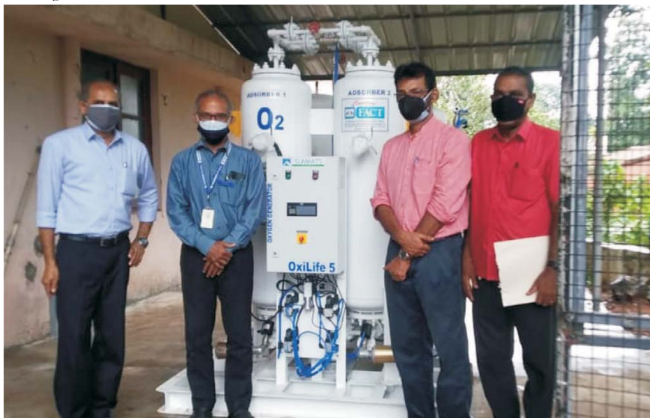
PSA Oxygen plant installed at PHC Ramamangalam.
