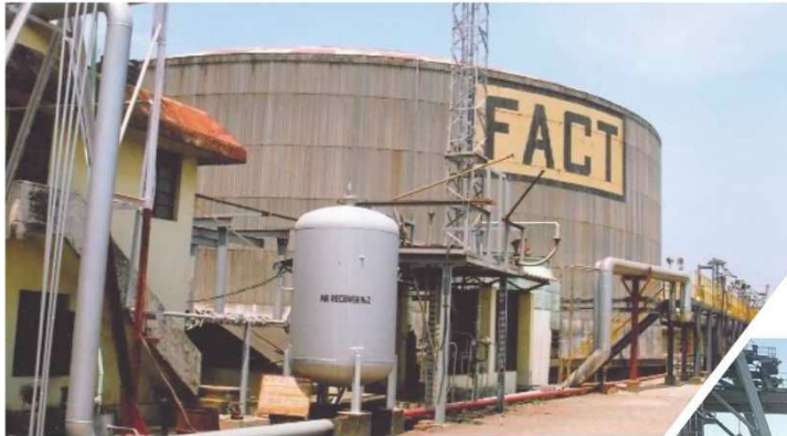
Ammonia Handling, Willingdon Island, Cochin
